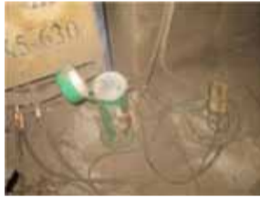
The "Bad" - uncontrolled welding
